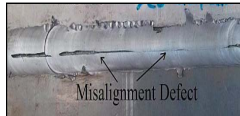
Fig.11. The misalignment of weld.
